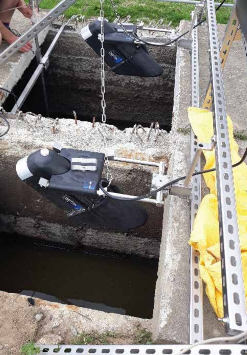
Figure 3. Laserflow Sensor Installations.
