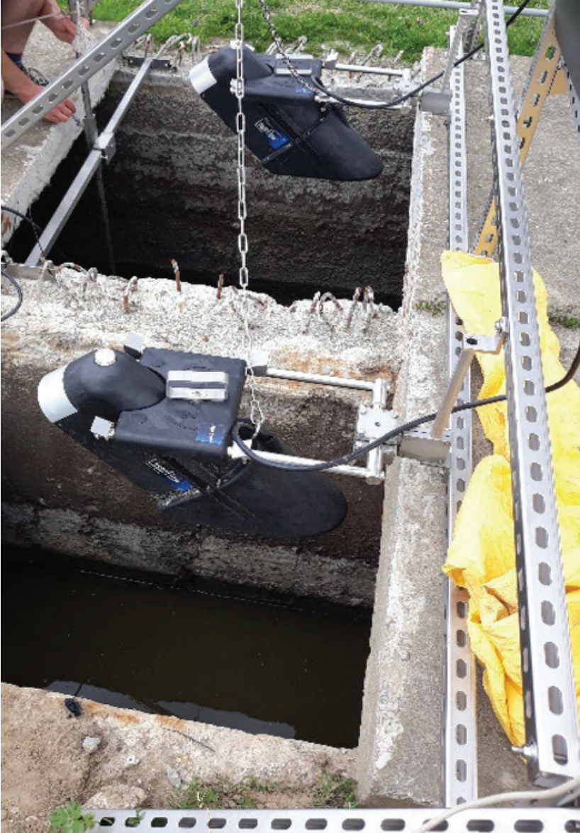
Figure 3. Laserflow Sensor Installations.
