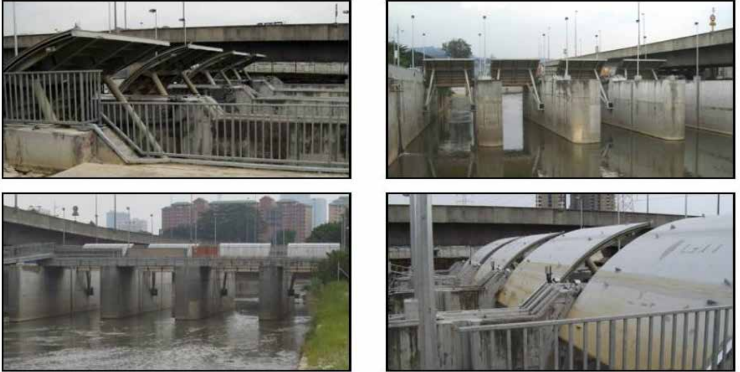
Figure 2. Radial Undershot Gates, controlled by the Flood Detection System, regulate flow to the City and into the tunnel.
