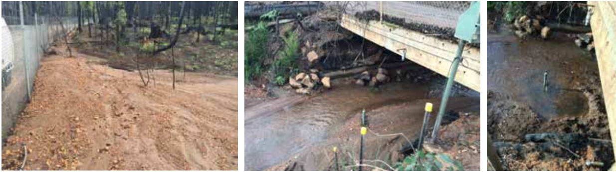
Figure 14: June 2016 (4 months after the fire) 6215W000 Samson Brook at Scarp Rd. Top Left: Hillslope Erosion, Centre: Sediment Build up in the channel, Right: Excavated pool around DO Sensor.
