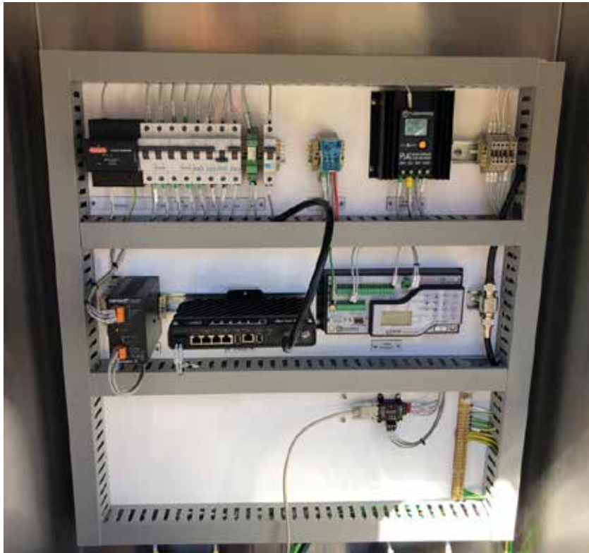
Figure 4: Station backing panel consisting of SCADA RTU, data logger, and solar system.
