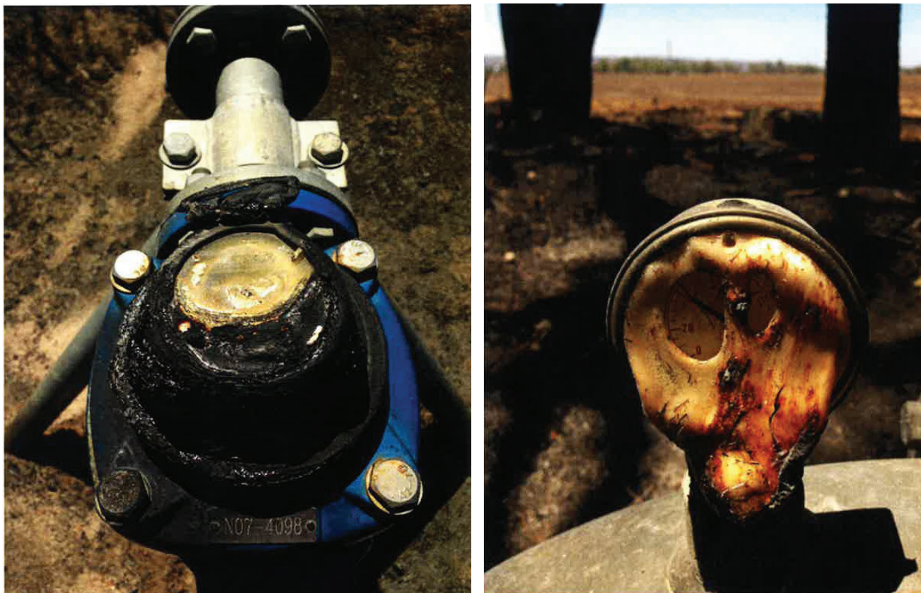
Figure 7: Example of Harvey Water Hydrometric Assets damaged by the Waroona Fire. Left: Mechanical Meter, Right: Pressure Gauge.
