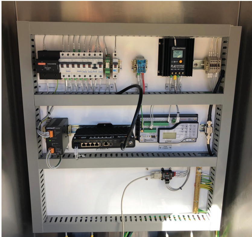
Figure 4: Station backing panel consisting of SCADA RTU, data logger, and solar system.
