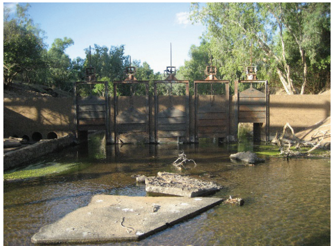
Figure 7: Offtake Gates to Uralla Creek.
