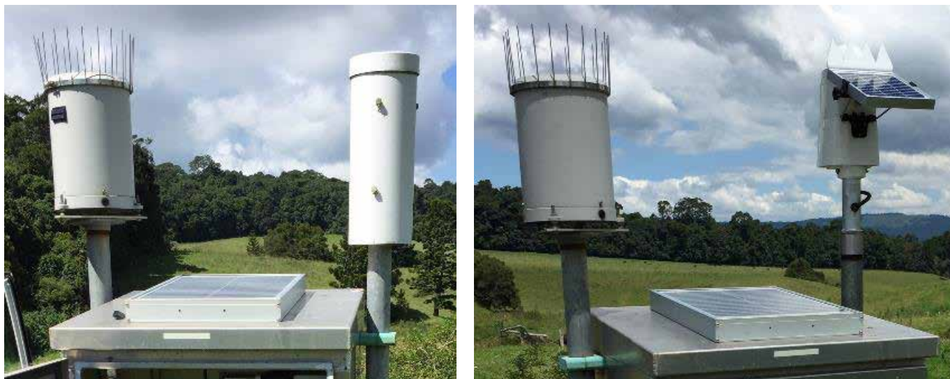
Figures 4 and 5. Before and after installation of SatVUE at Globalstar telemetry site.
