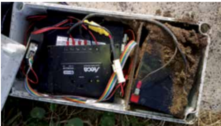
Figure 5. Image shows an accumulation of dirt from an ant's colony that has disrupted the external modem unit at a sewer monitoring site.
