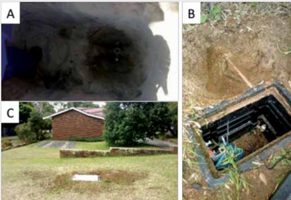
Figure 2. Process of Installing a Pressure Recording Gauge; A) Tapping into a water main, B) Connecting copper piping from the main to a ballvalve to a PRG inside a constructed pit, C) Finished PRG underground monitoring site.
