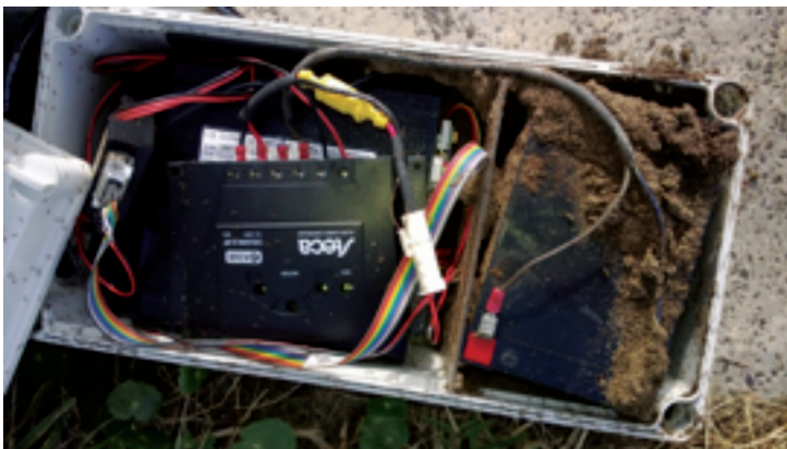
Figure 5. Image shows an accumulation of dirt from an ant's colony that has disrupted the external modem unit at a sewer monitoring site.
