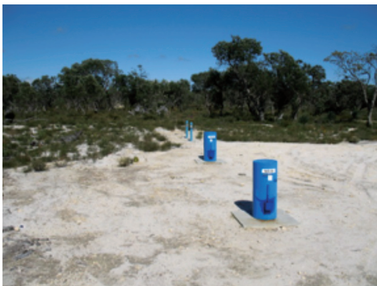
NG3 Site prior to installation of IP Telemetry.
