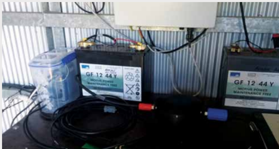
DL25 logger set up in gauging station hut.
