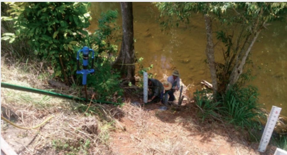
Juan Bouttell and Daryl Harper helping with the installation of the HADCP.
