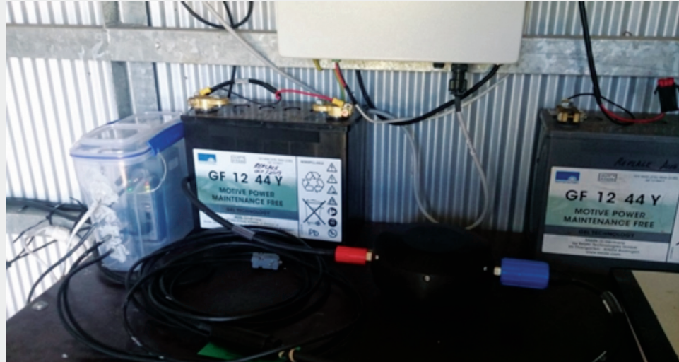
DL25 logger set up in gauging station hut.
