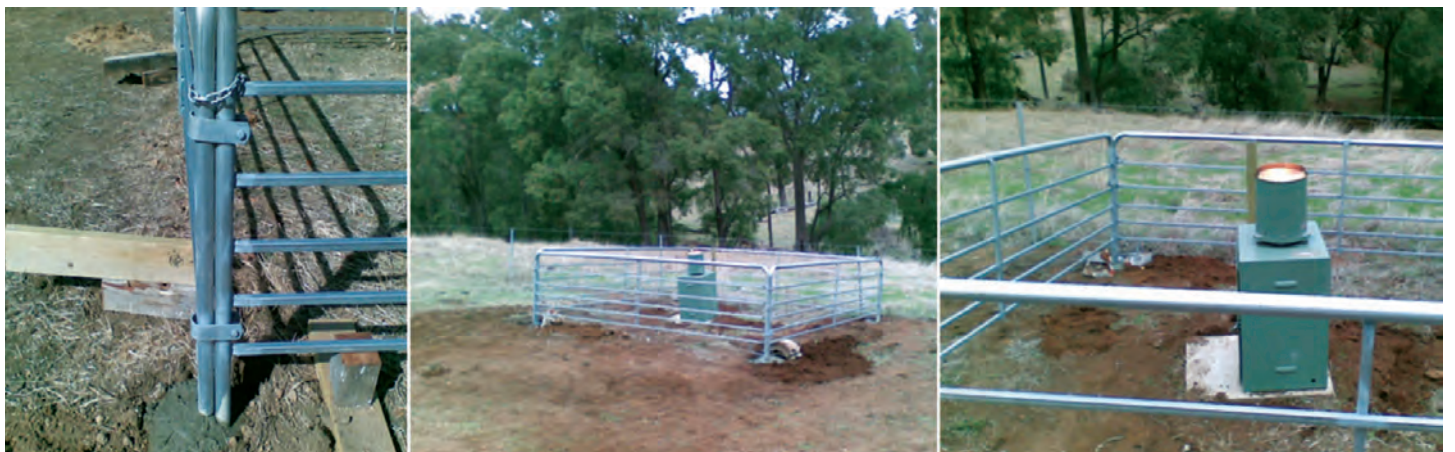
Left: Close up view of the hinging and corner brackets at George Road pluvio. Middle, Right: Sandalwood site constructed on sloping ground.
