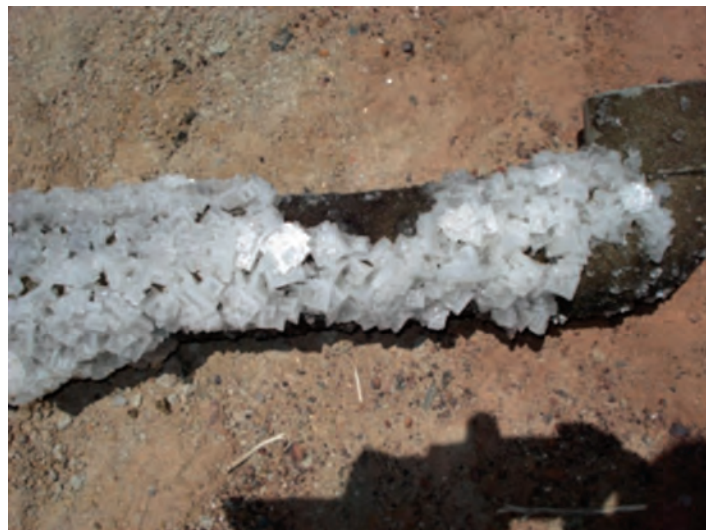
A section of inlet pipe covered in crystals.
