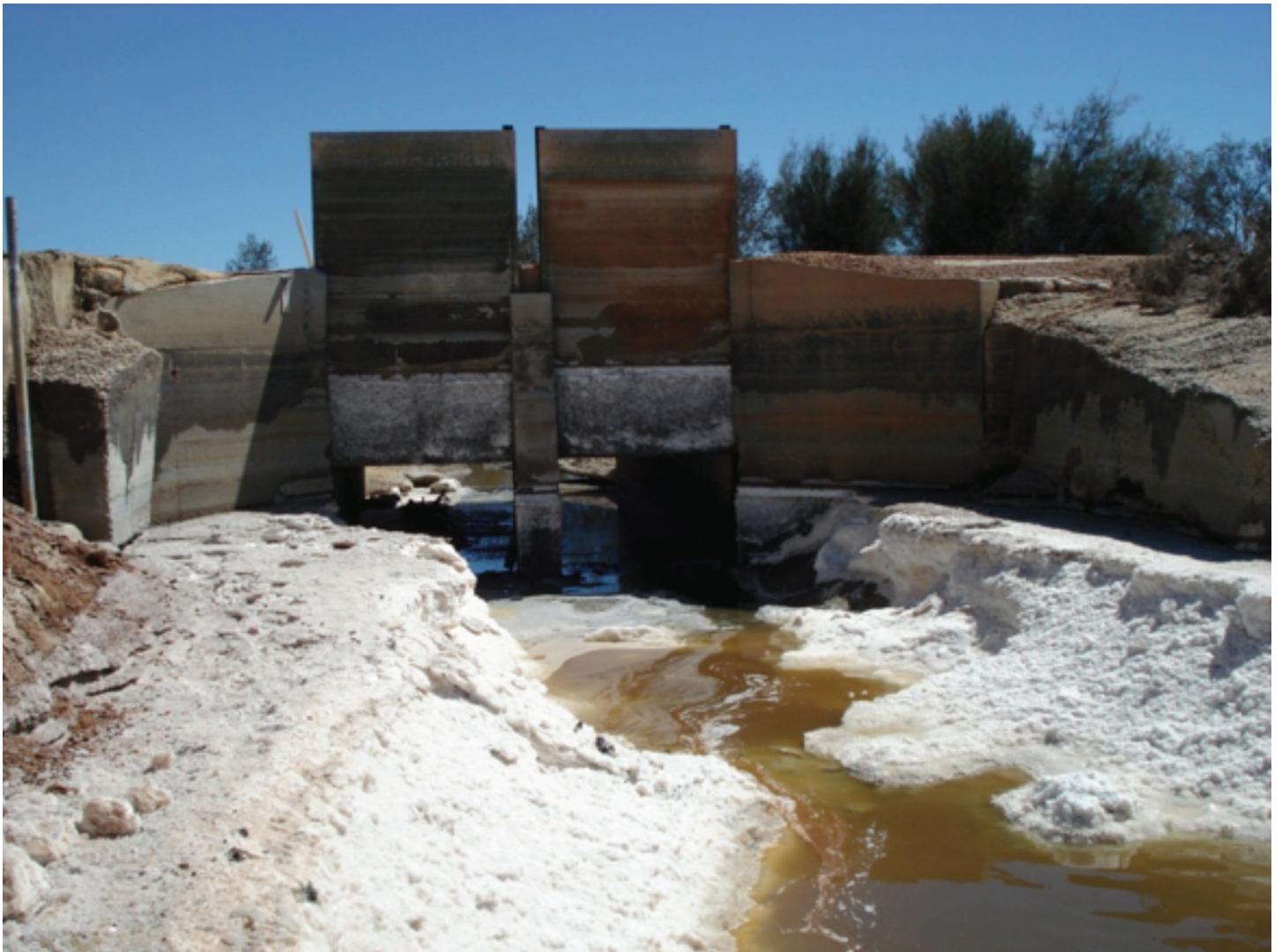
Gates (open in the picture) controlling water releases into the Avon River. (Yes, that's salt on the banks, and that is after much of it had been flushed away.)
