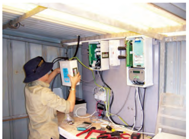
Another Neon install at Emu Springs.
