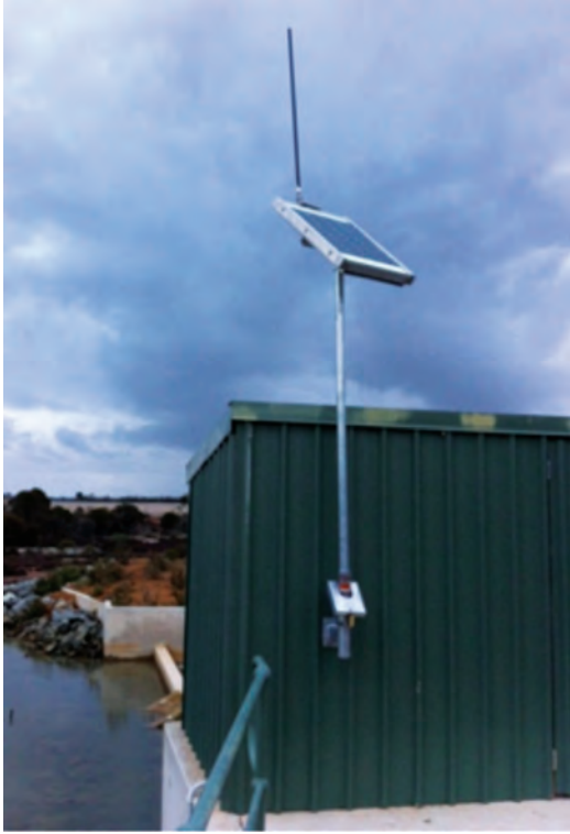
Full system installed with security cover.
