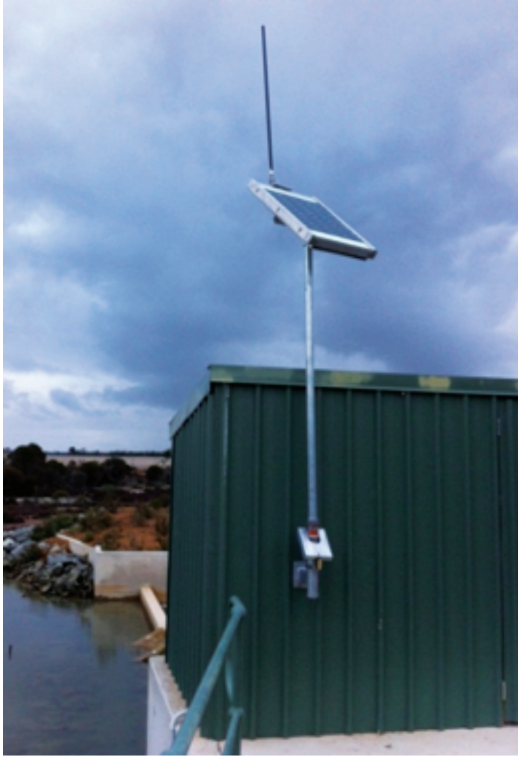
Full system installed with security cover.
