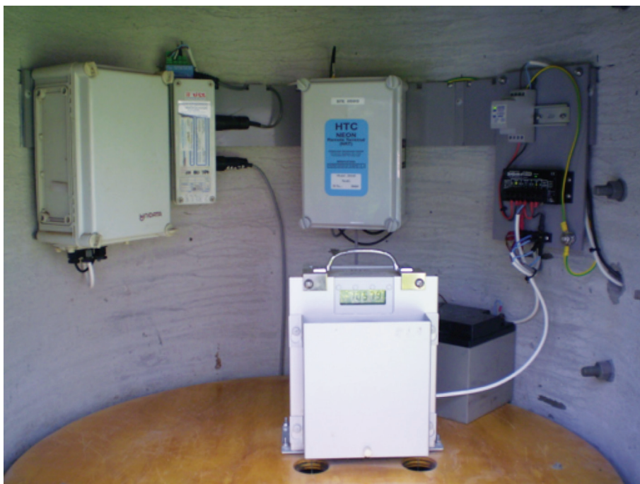
Completed Neon instrumentation layout.
