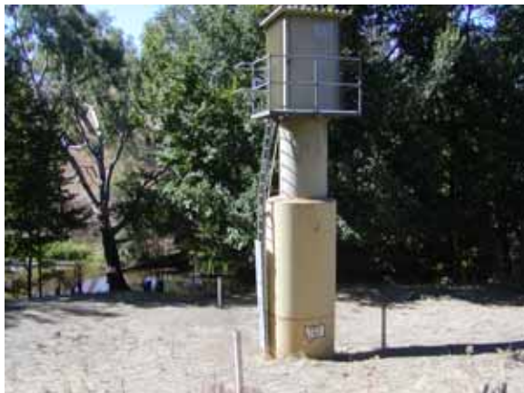
Photograph 3 A 1970's float well installation.
