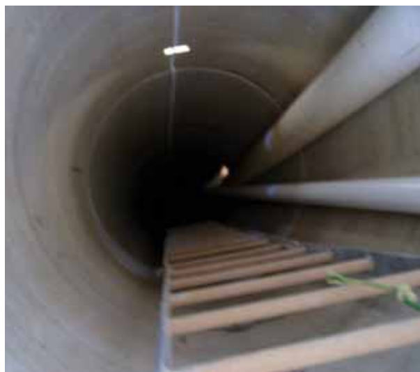
Photograph 4 - The inside of a float well.
