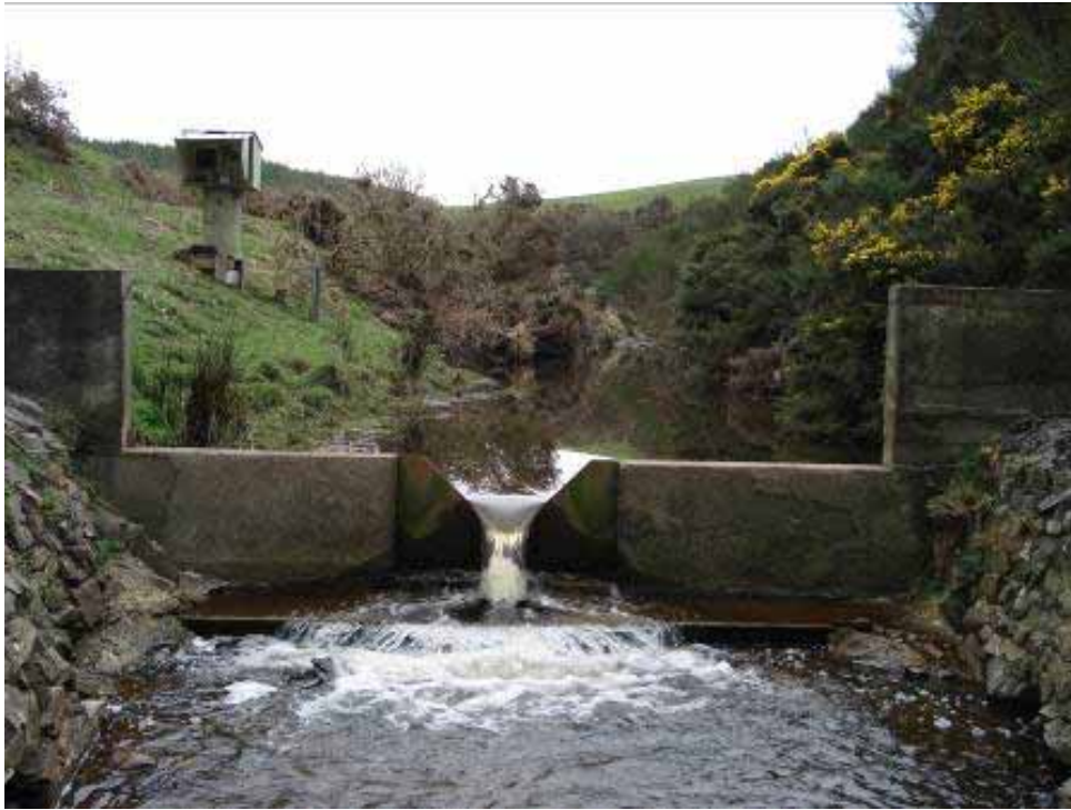
Figure 6: The weir and flow recorder at Nobles Stream at Bull Creek Road (site 74701).
