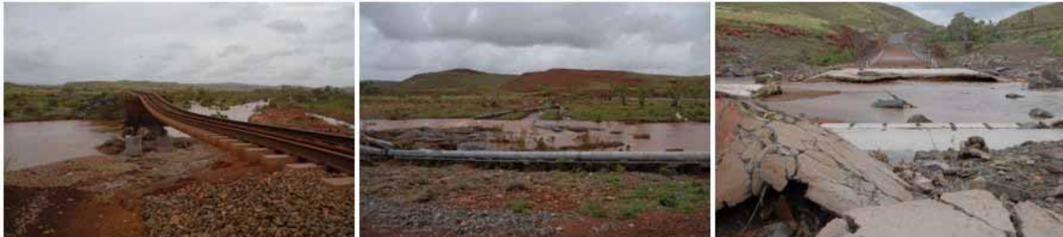
Flood damage in the Pilbara
