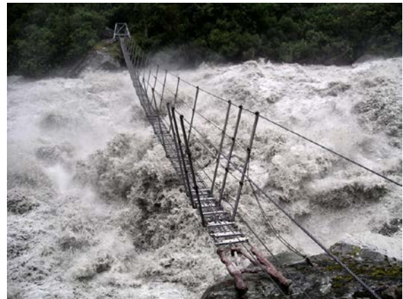
Upper Wanganui River (South Island) in flood 2004
