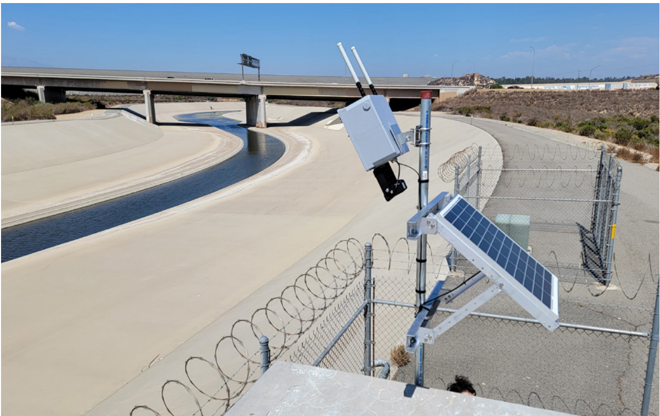
Figure 3: CVSG system installed at USGS gaging station 1107400, Santa Ana R BL Prado Dam, CA.
