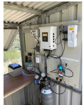
Gas Pressure Instrumentation
